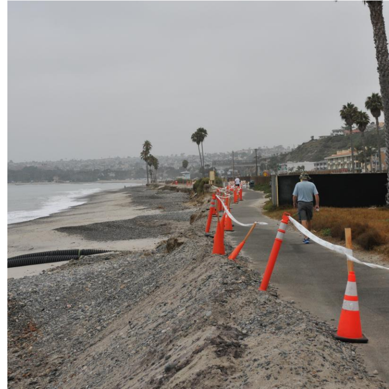
Impacts to bike path and exposed drainage pipes on beach
