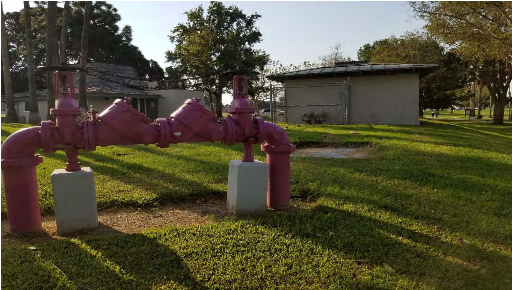
Photo 7 – Pump house and associated infrastructure. Ranger station can be seen in the background to the left. Southern portion of site. Looking south.
